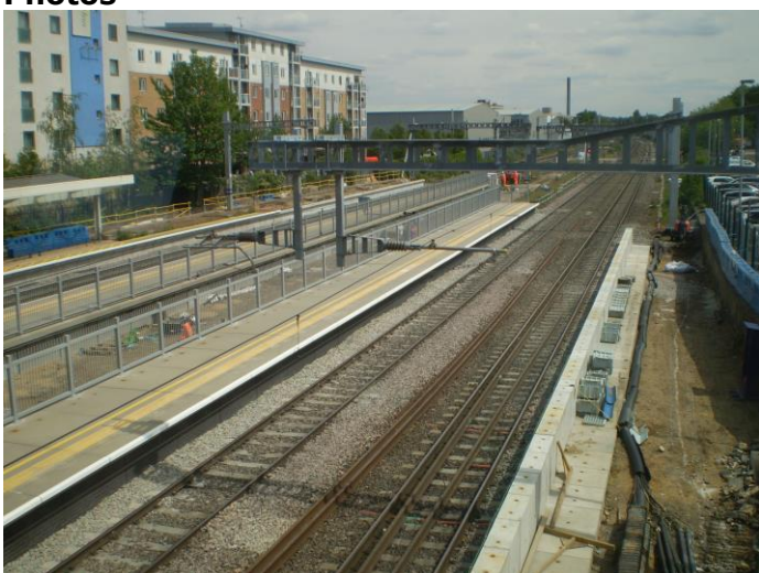
Platform extensions being built at the east end of Slough station, seen on 22 nd May 2019.
