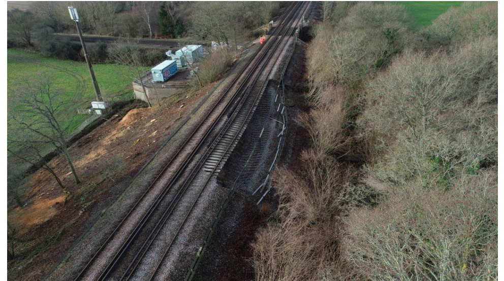
Tonbridge – Reigate Landslip – December 2019
