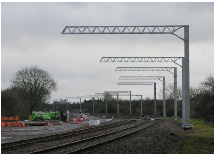
Up a gantry. Overhead support masts and cantilevers installed at Braybrooke, just south of Market Harborough, over the Christmas break. Good progress is being made with the electrification from Kettering.
