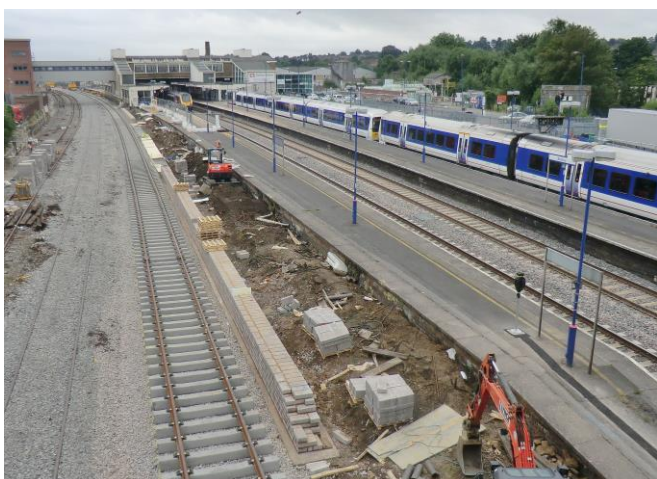
The new up through platform and loop under construction at Banbury, July 2016.
