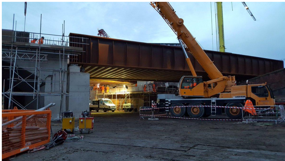
The new bridge over Water Street in Salford that will form part of the Ordsall chord linking Manchester's Victoria and Piccadilly stations directly for the first time. This work will form part of infrastructure that will require new/additional trains. Photo courtesy Network Rail.
