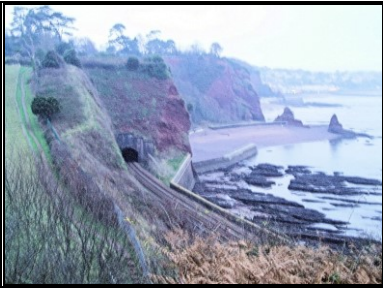
Above. Steep high cliffs between Parson's Tunnel and Clerk's Tunnel to north in view. The rock is competent (strong) so unlikely to slip, but small rock falls are a potential hazard.
