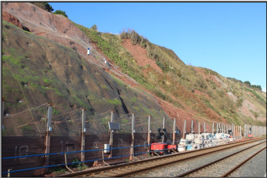
Site of the Woodlands Avenue landslip of February – March 2014 on 7 November 2014. Photo by Geof Sheppard , Creative Commons Attribution-Share Alike 3.0 Unported licence .
