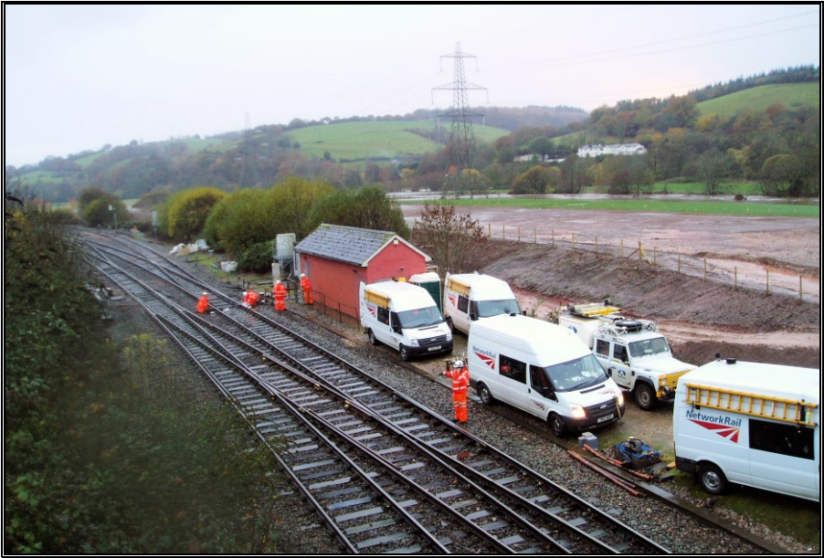
Network Rail busy on the tracks leading up to Cowley Bridge Junction on 22 nd November 2016.
