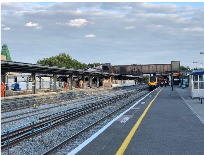
Platform 4 was open for 5 days, southbound only, while the others were resurfaced and track through the station was re-laid.
