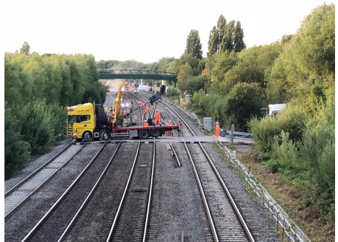
An old signal is removed between Walton Well Road and Aristotle Lane.
