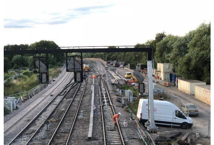
The new up line from Oxford Parkway is connected to the Up Oxford Relief line seen from Aristotle Lane. All: Richard Stow
