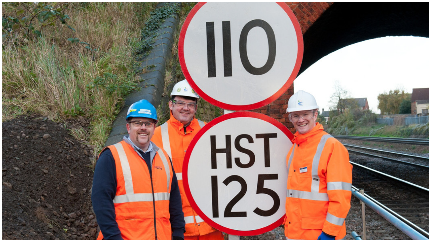
New 125 speed limit signs being installed at Bromham Road bridge, Bedford. From left, are Richard Walker, the route delivery director (East Midlands) for Network Rail, Dave Diskin, the framework manager from contractor Carillion and David Horne, managing director for East Midlands Trains Picture: East Midlands Trains
