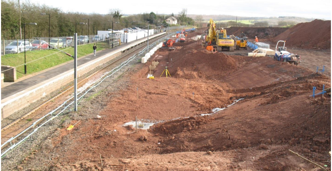
Working towards double track and the second platform - adjacent to and west of the existing platform
