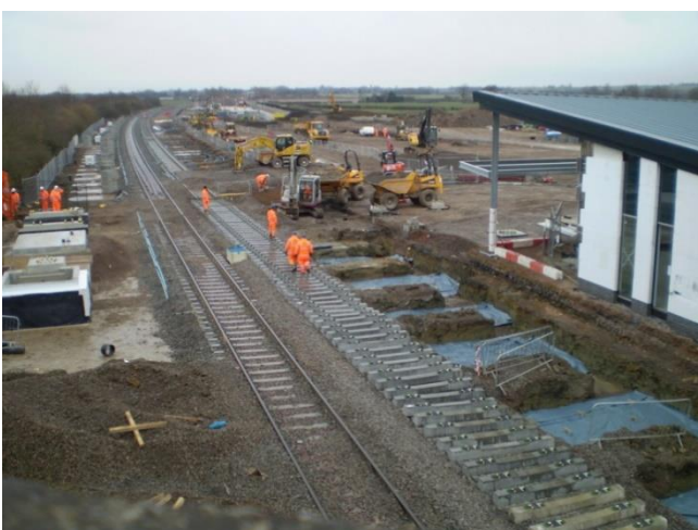
View west at Bicester Town showing new MOD junction. Islip station site showing new platform foundations.
