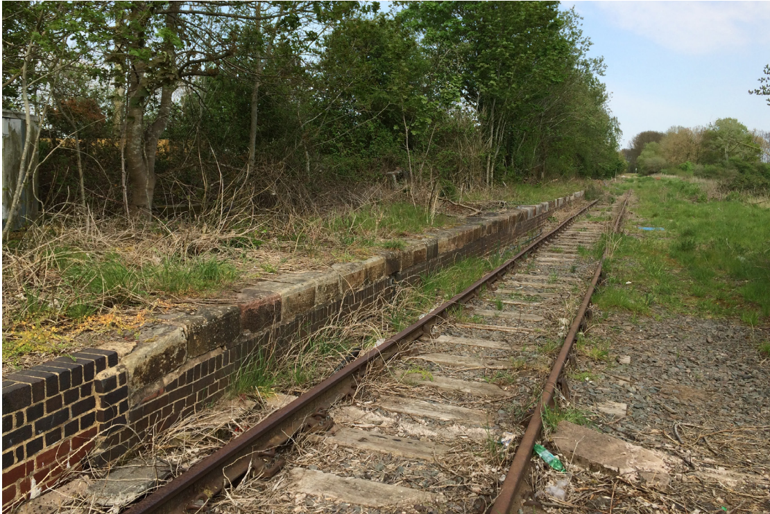
STOP THE ROT: The Oxford-Bletchley line near Steeple Claydon in 2016
