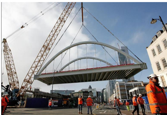
East London line to the left, Broad Street viaduct to the right
