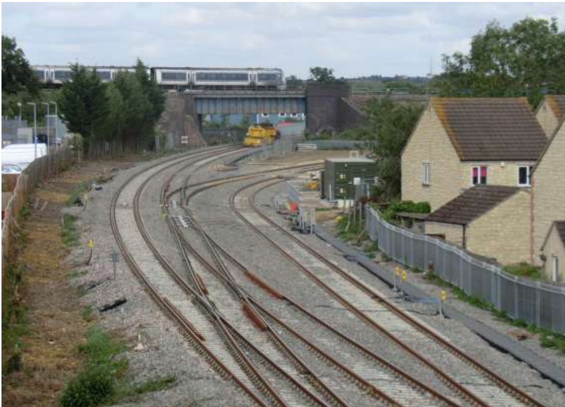
(above) Bicester Gavray Junction showing the new link to the Chiltern main line while EWR will continue under the bridge where the road-railer machine is stabled in a short siding. 3 August 2015
