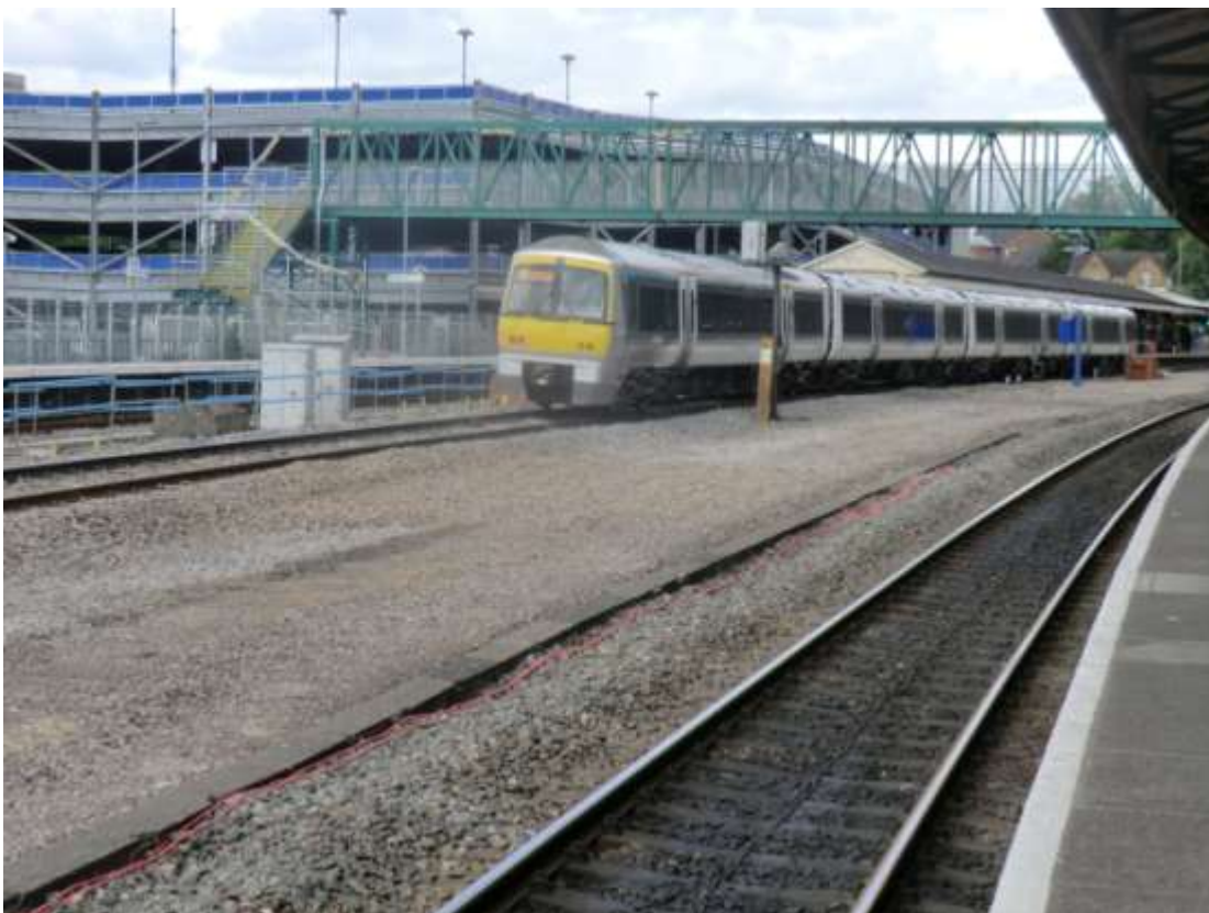
Showing temporary footbridge while the down platform is lengthened to take 9-cars at Wycombe as the 12:15 MYB to Birmingham passes through on 17/07/15. A 2-storey extension to car park is planned.
