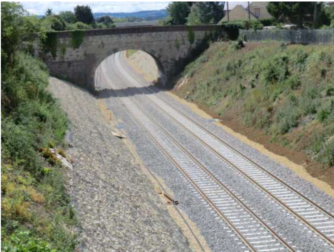
Double track is now complete and fully connected between Bicester South Junction and Oxford Parkway. Shown here in the previously waterlogged cutting at Islip 19/07/15
